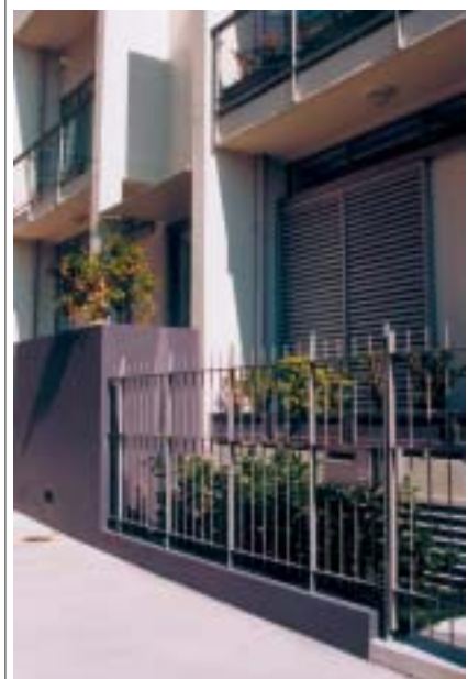
Street level picket fencing with planting provides screening to car park ventilation louvres.
