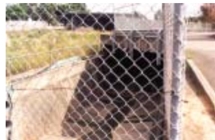
A'Beckett's creek, water flowing through an open culvert on the Rositano site.
